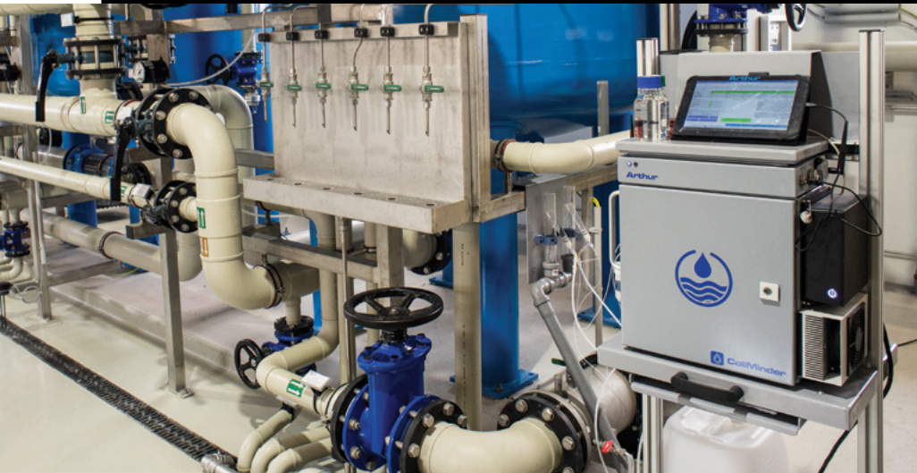
ColiMinder Arthur monitoring drinking water production in a municipal drinking water plant
