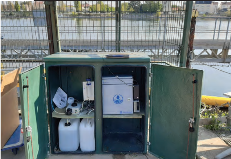
Left: The ColiMinder "Arthur" monitors the Seine's water to detect probable CSOs from wastewater treatment plants upstream
